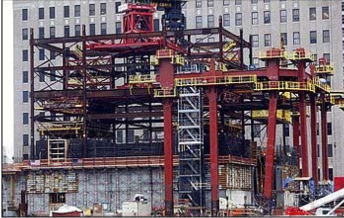
The base of the Freedom Tower is seen under construction at the World Trade Center site in New York on Sept. 11 of this year. (By Chip East -- Associated Press)
